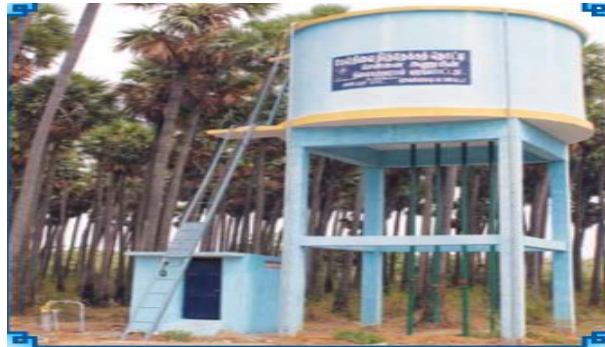
New Water Tank 60,000 litre Capacity along with Bore well and Pump Room Executed by MAPS at Kadambadi Village
