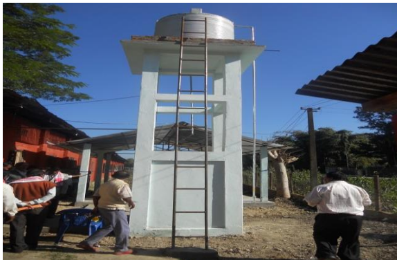
Over Head Tank & Laying pipe line for drinking facility to Bhadoi High School at Bhadoipanchali, Assam.
