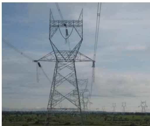
High Voltage Transmission Lines to conserve Natural Resources
