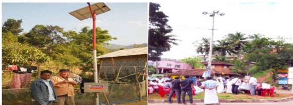
Solar Lights and LED Street Lights
